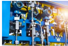
Motor heating Control
